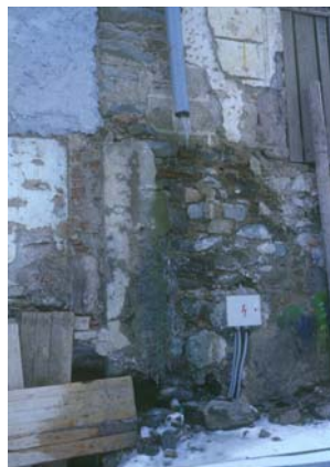
More than 20 years missing downpipe is continuously damaging walls, foundations and ground soil. - House on The Trinity square – Banska Stiavnica
