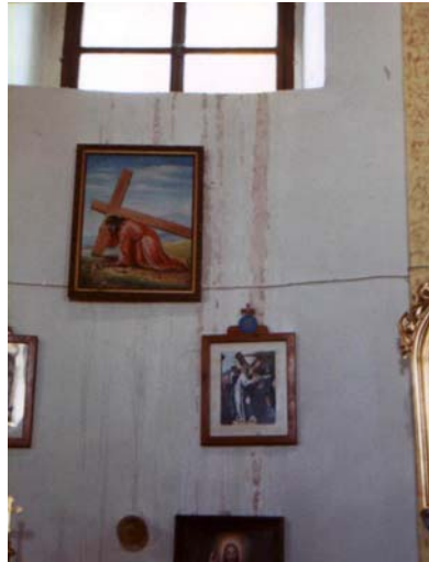
Water condensation on the window glass sheet causes damage to painting, plaster, and to window frames as well. - Greek-catholic church of Virgin Mary in Chmelova
