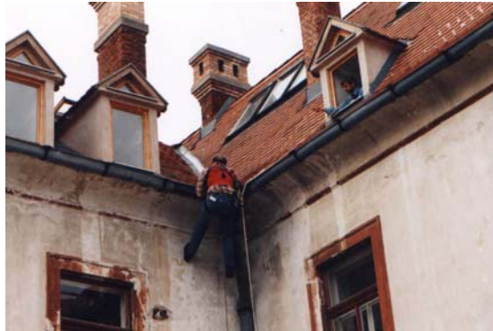
Inspectors beside preparing reports can provide „first aid“ repairs - Team of Monumentenwacht Netherlands inspects Palffy's manor house in Svaty Jur.
