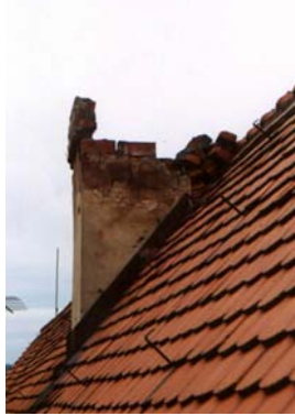
Bricks falling from the top of chimney are dangerous for roofcover. - House No. 38 on The Town Hall square – Bardejov
