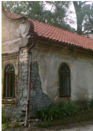
Although there were some maintenance activity done, they are not sufficient since they were related to consequence not to cause of the damage. - Garden house of the castle at Liblice
