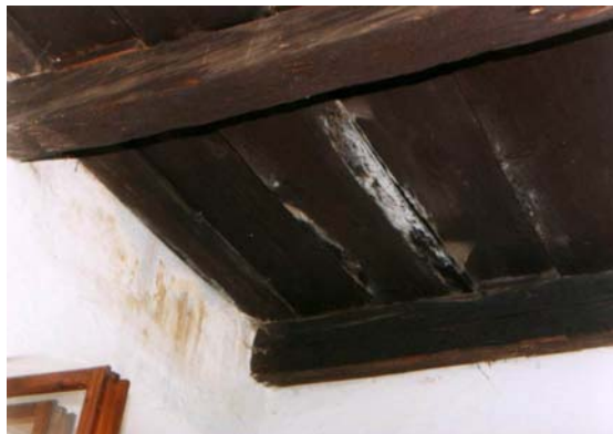
Mould on the wooden ceiling indicates high humidity above the ceiling. - Building on Town Hall square 3A, Bardejov
