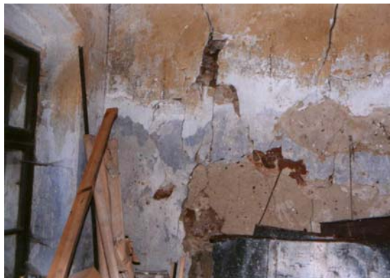
Cracks on the wall occurred during construction works on neighbouring house. Although they are not moving any more, they must be maintained, not to cause more damage. - Jewish synagogue on Klastorska street – Bardejov
