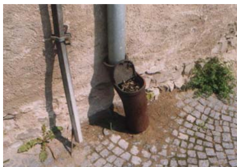
Very simple activity – cleaning certain points on drainage system - can avoid many problems. - House in Town reserve Litomerice
