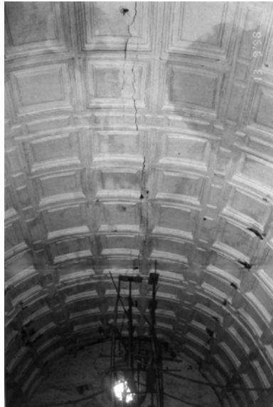
Figure 2: Interior view of the Nave vault – showing the crack
