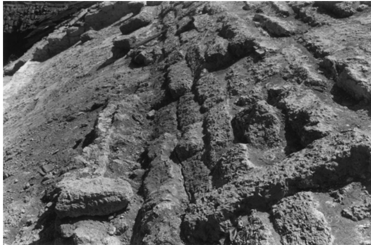
Figure 6: Photograph showing the vault surface when exposed with the timber roof dismantled
