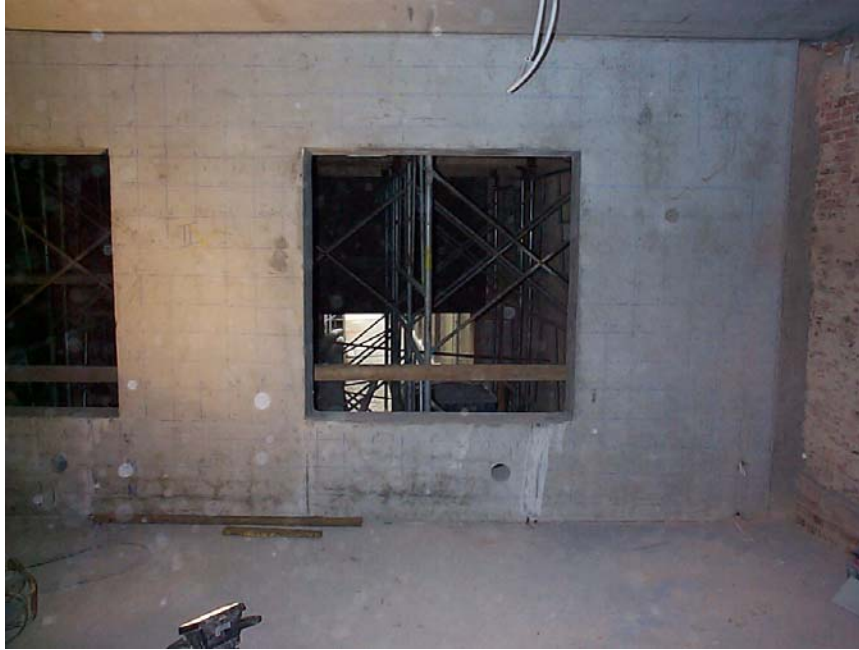
Fig. 1: The investigated wall consists of two prefabricated faces filled up with poured concrete. The raster shows the measuring points.
