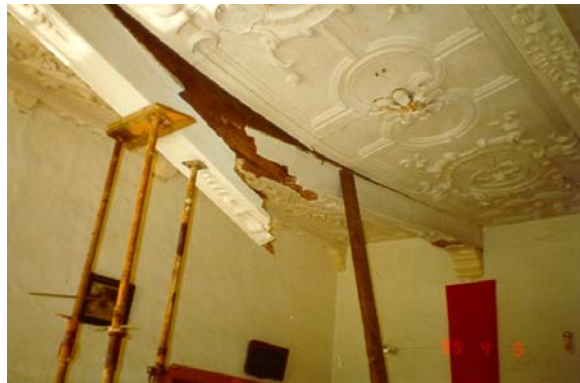
Fig. 14: The wooden beam broke due to overloading and deterioration
